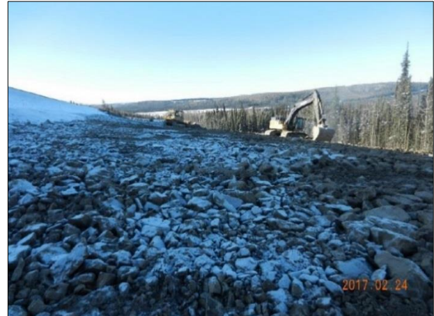
Figure 11. View of rockfill buttress construction in late February 2017, looking west towards Pink Mountain. Note tracked equipment in the middle of the photo for scale.
