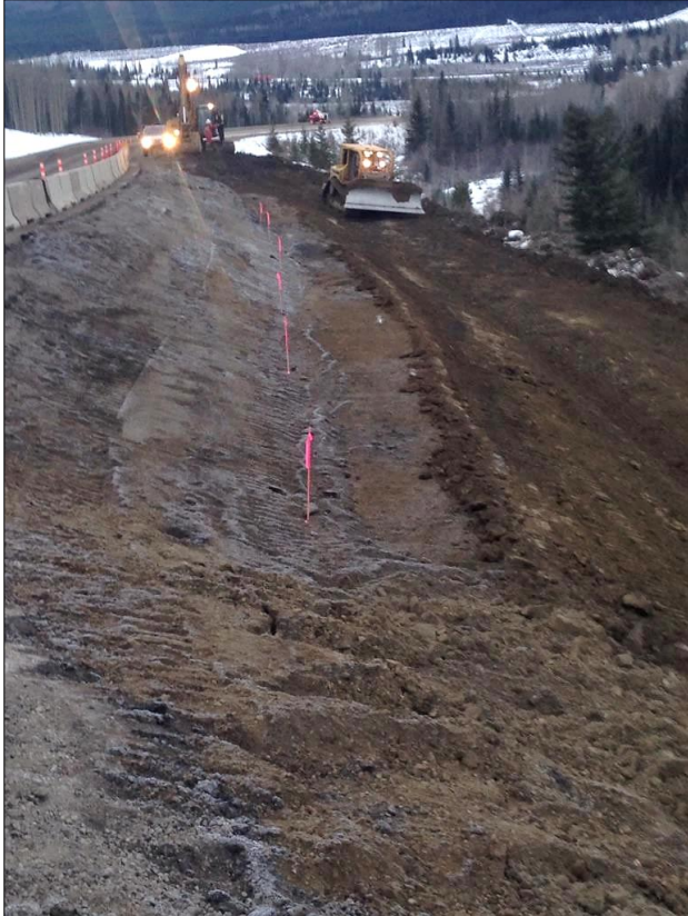
Figure 8. View of emergency unloading work (embankment removal) in early November 2016, looking west towards Pink Mountain.
