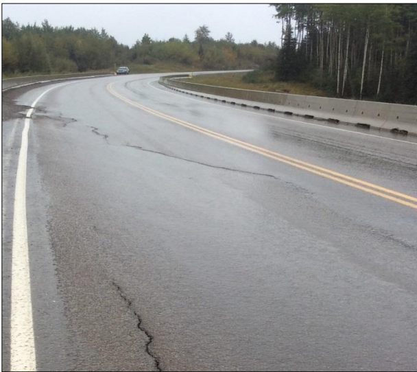
Figure 3. View of km 201.4 slide area in early September 2016, looking down-chainage (east) towards Fort St John. The parked vehicle is located at about the transition point to the bedrock through-cut section further to the east.
