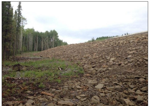
Figure 12. View of the completed rockfill buttress in early August 2017, looking east towards Fort St John.
