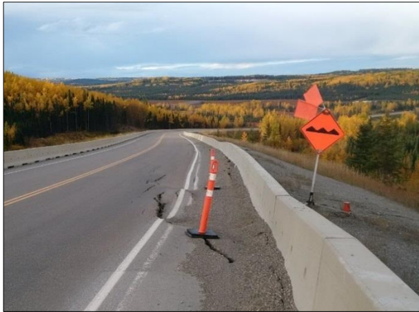
Figure 2. View of km 201.4 slide area in mid-September 2016, looking up-chainage (west) towards Pink Mountain.
