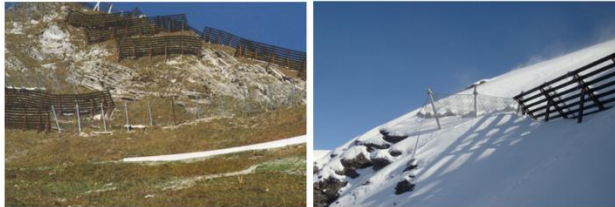
Figure 4. Rigid steel snow-bridges and flexible snow nets side by side
