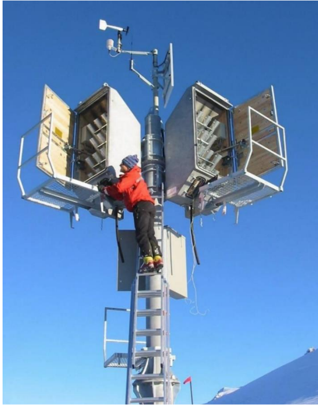
Figure 16. Avalanche Guard RACS system. As of 2016, there are six of these systems installed at Fortitude and Fidelity/Park One avalanche paths near Rogers Pass (photo courtesy of BC Ministry of Transportation and Infrastructure)
