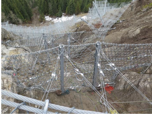
Figure 13. Use of Debris Flow net barrier in CC7 gully
