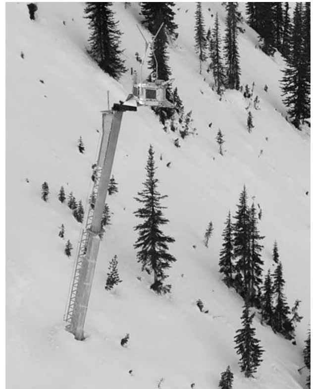
Figure 15. Wyssen Tower explosives-based RACS. This Wyssen Tower system was installed at Cutbank during summer 2017
