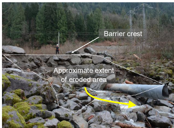
Figure 4: Looking upstream at the partially reconstructed Patterson Creek barrier following overtopping during the November 2017 event. Photo by J. Park, December 2017.
