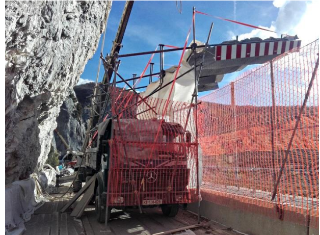
Figure 5. Cantilevered screen to protect traffic from drilling operations. Wooden planks used to protect the road surface can also be seen.
