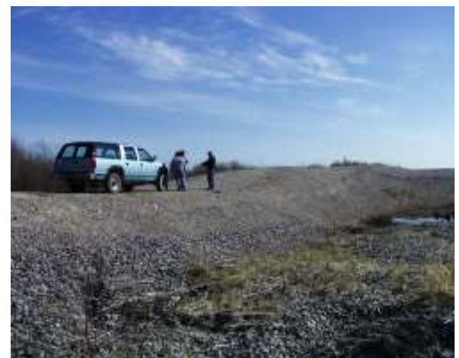
Example of differential settlement along a section of dike prior to rehabilitation.
